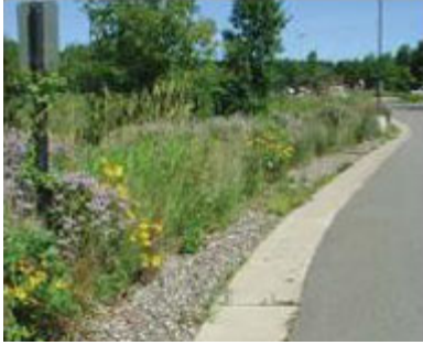
Example of Infiltration Practices Infiltration trench, Lino Lakes City Hall — Link Lakes, MN
