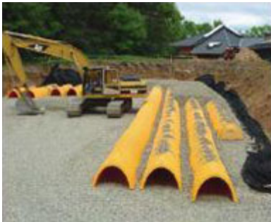
Example of Infiltration Practices Underground storage and infiltration, Bradshaw Celebration of Life Center — Stillwater, MN
