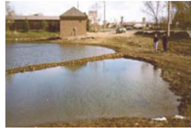
Example of Chemical and Biological Treatment Tanners Lake alum injection facility — Oakdale, MN
